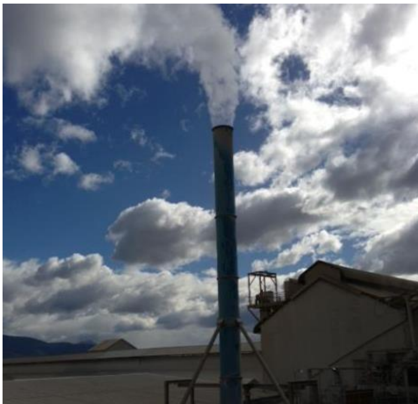
Broadfield Mixer Scrubber Stack (Den Stack)
