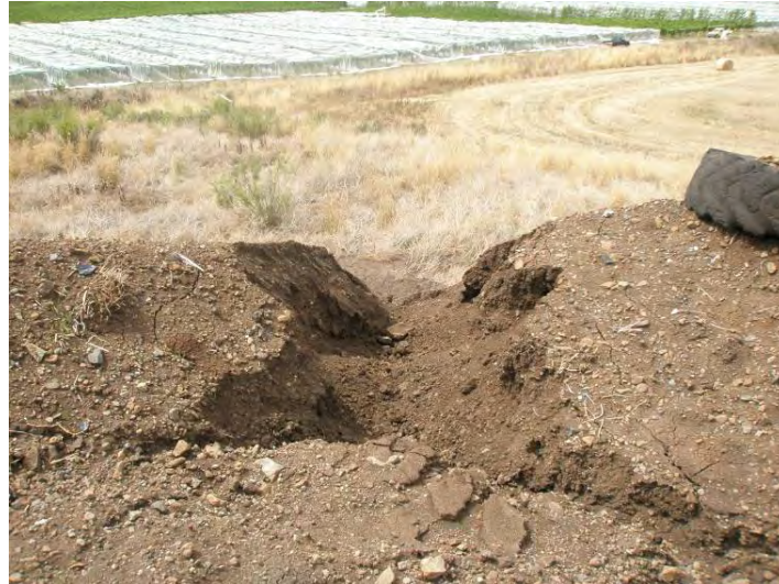
Plate 6 : East facing batter erosion as a result of concentrated discharge
